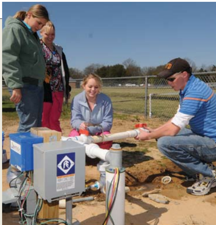
McBee High Students got some hands-on learning as a result of the creativity of their instructor, Pat Earle, and a grant from The Byerly Foundation, which helped them design and install an irrigation system for a ball field.
